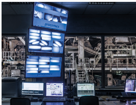
KM6 control room
